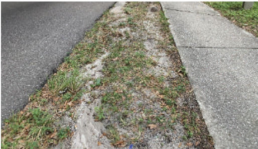
Figure 2-13 - 2919 E Sligh Avenue Erosion
