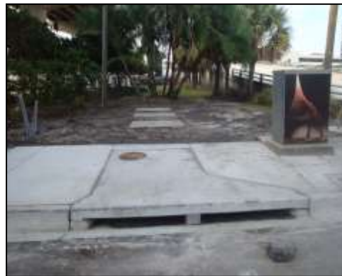
Stormwater scrubbers filter water and capture waste before water enters the Hillsborough River and Hillsborough Bay.
