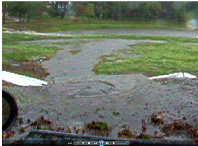
Picture No. 2 - Lake Roberta Manhole at Outfall Structure flooding on July 21 st , 2007
