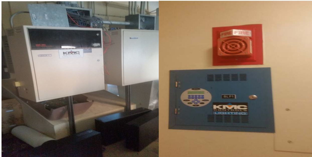
Examples of KMC Controls throughout building
