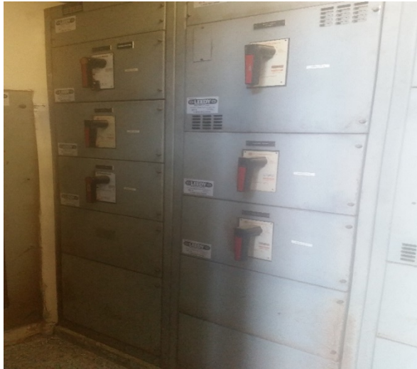
Electrical switchboard – 1 st floor TMOB
