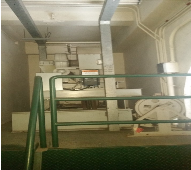
Elevator equipment at 9 th Floor mezzanine.
