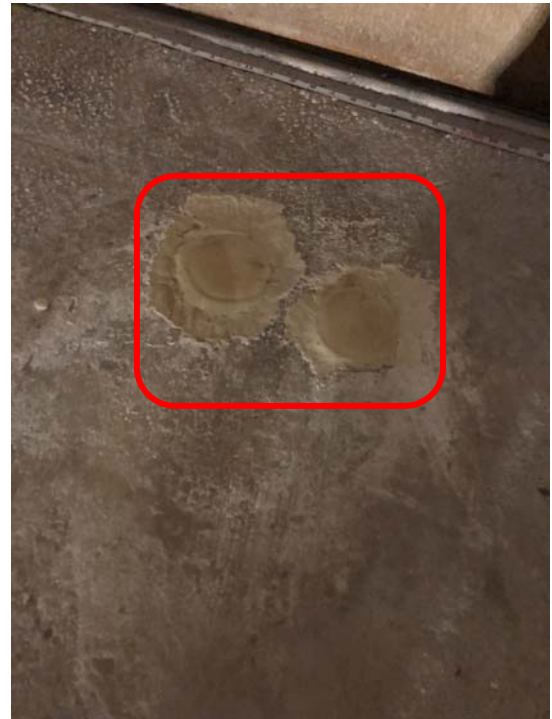
Site Picture 2 Showing Patches on the Tank Floor Slab
