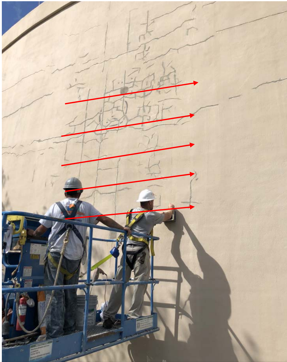
Site Picture 4 Showing the Survey Area of the Exterior Tank Wall and the Approximate Locations of the GPR Transects
