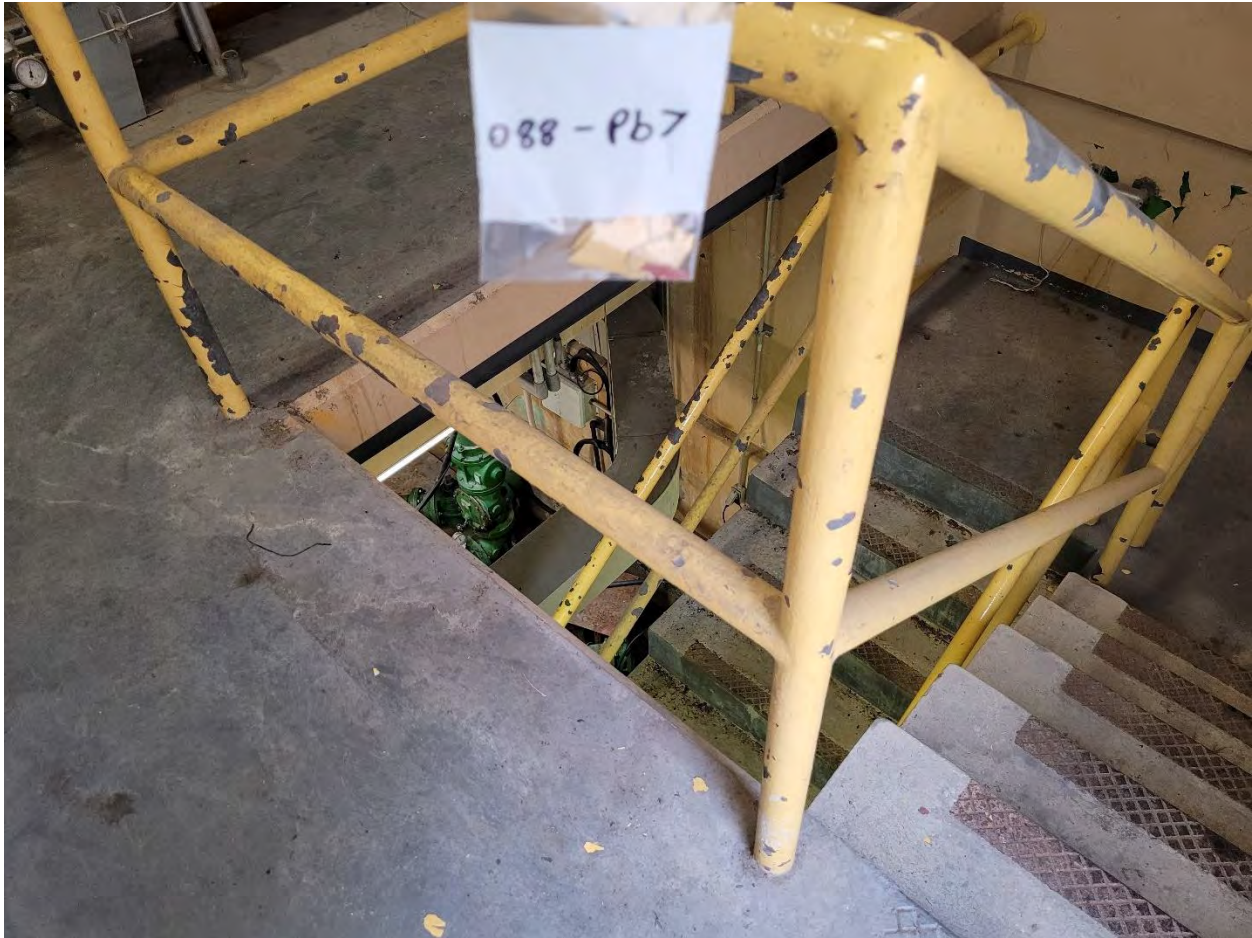
088-PB 7: Yellow w/ Red Paint on Metal Handrails [3.1 % wt]
