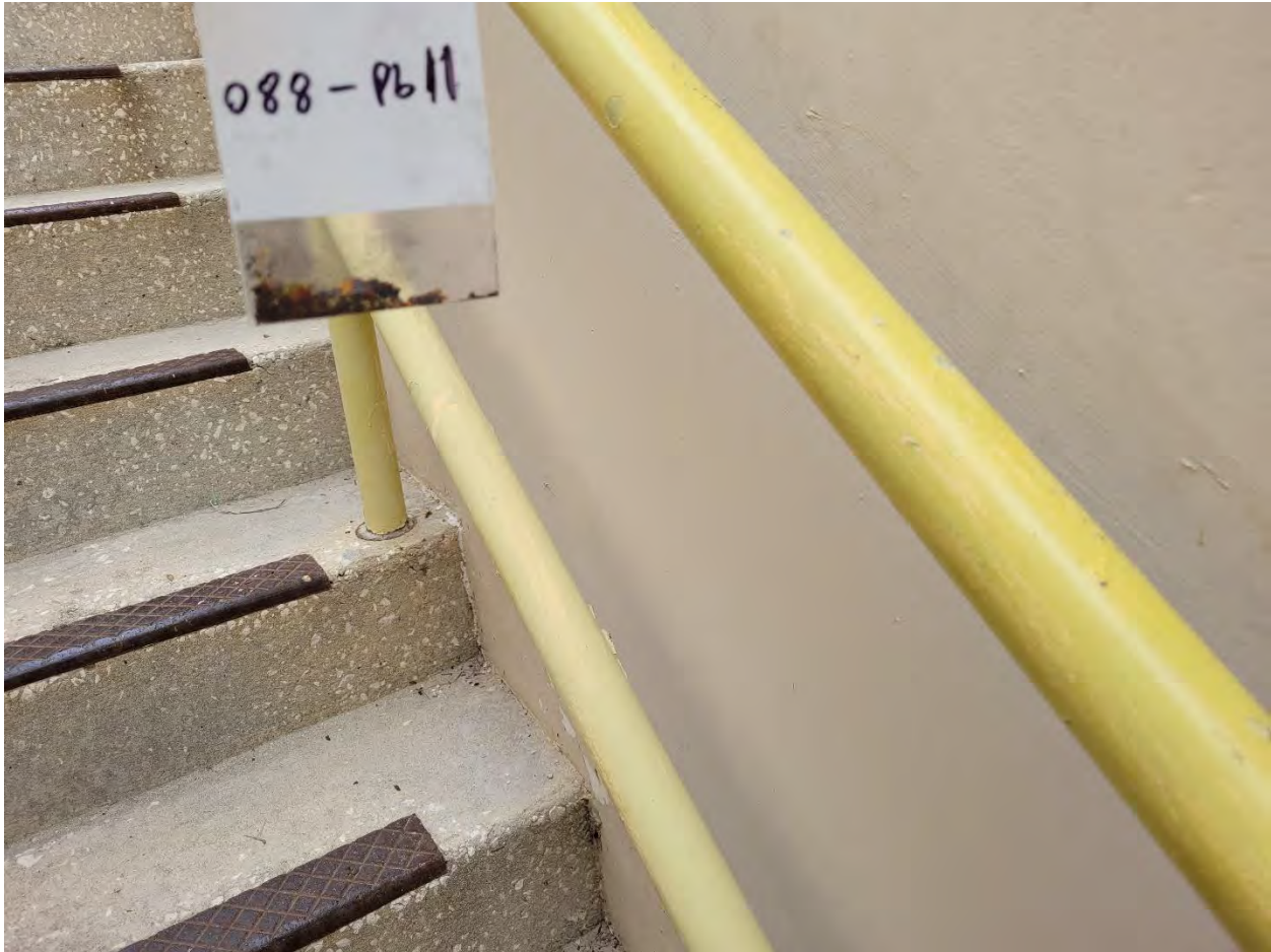
088-PB 11: Yellow w/ Red Paint on Metal Handrails [0.26 % wt]
