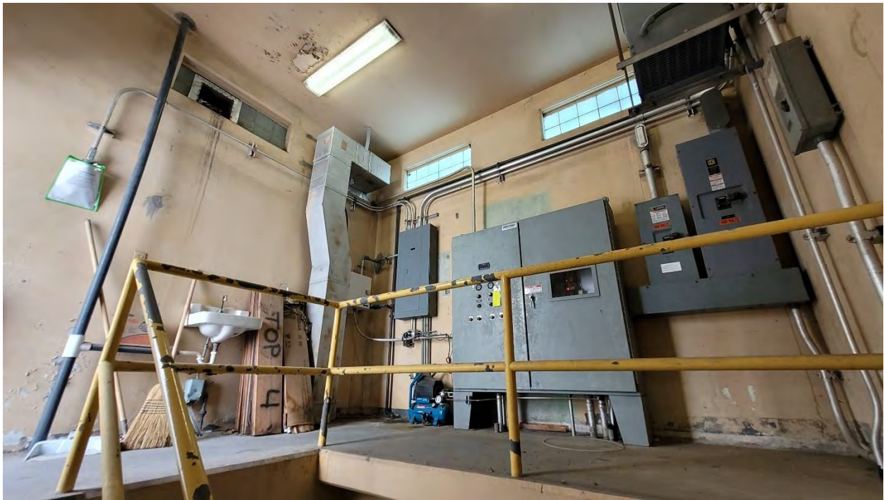
Electrical Panels and Ductwork should be sampled after the site is inactive
