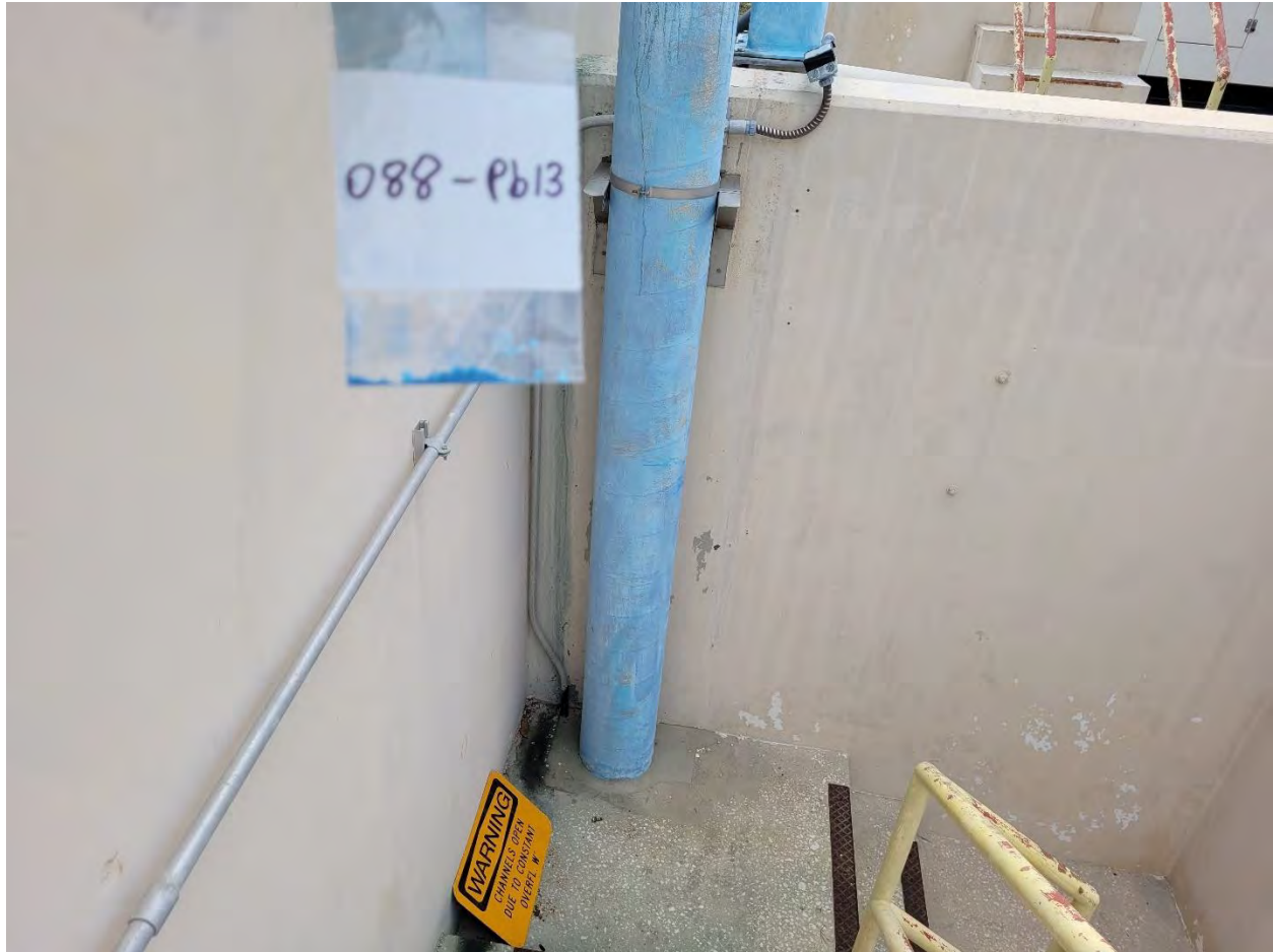
088-PB 13: Blue Paint on Metal Pipe [NLD]
