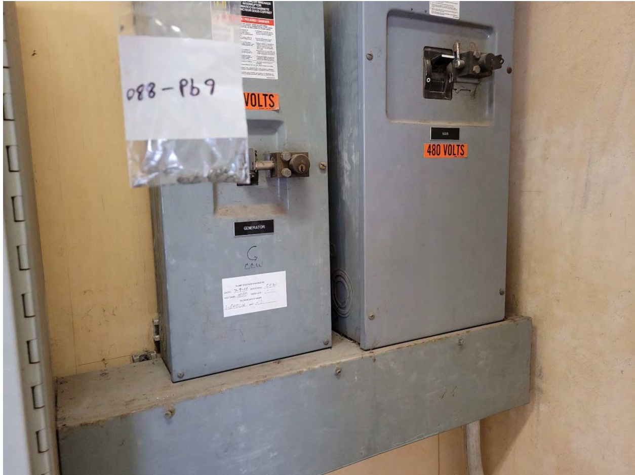
088-PB 9: Dark Grey Paint on Metal Breaker Box [NLD]
