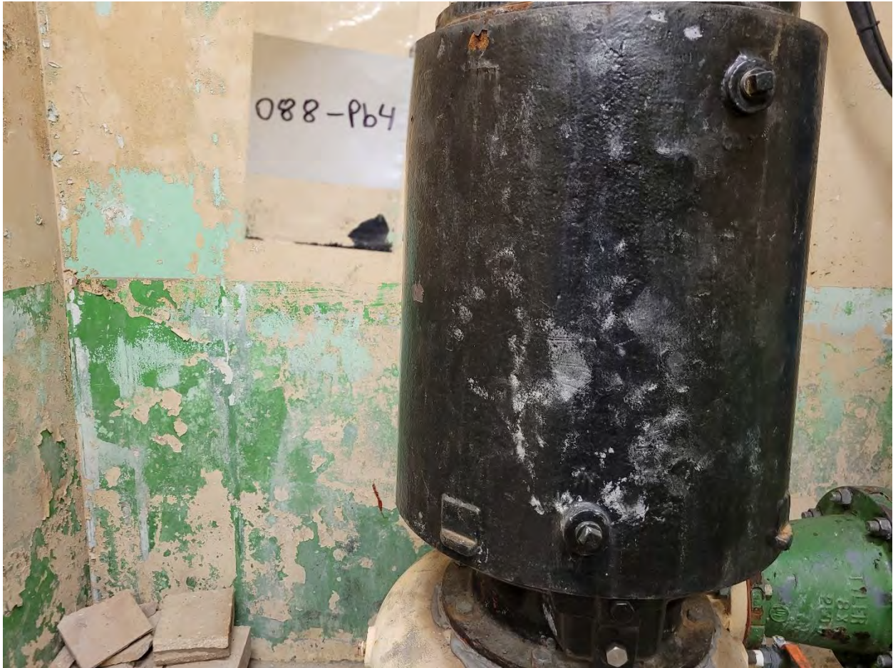
088-PB 4: Black Paint on Metal Pump [NLD]
