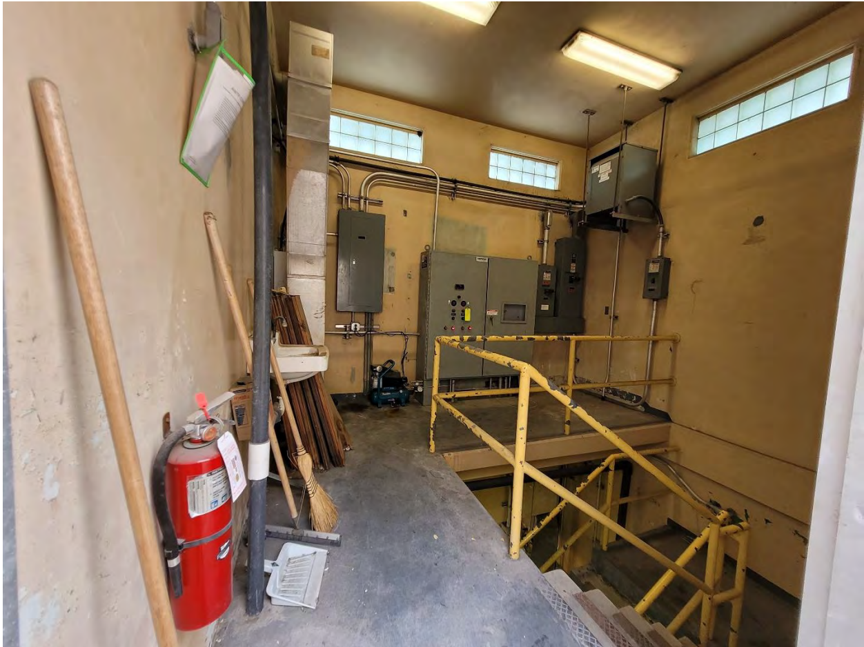
Pumpstation 192: Drywell, Level 1
