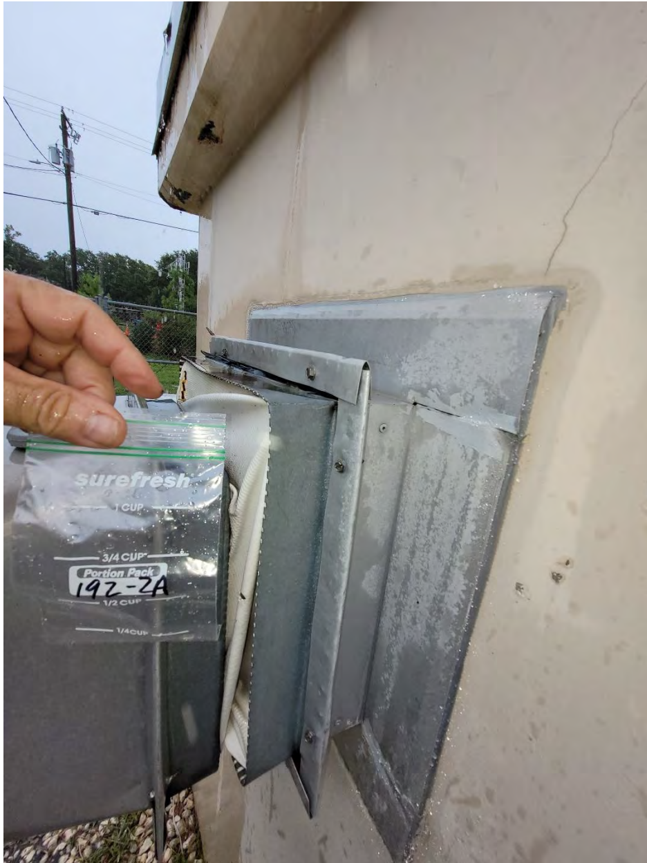
192-2A: HVAC Vibration Damper [NAD]
