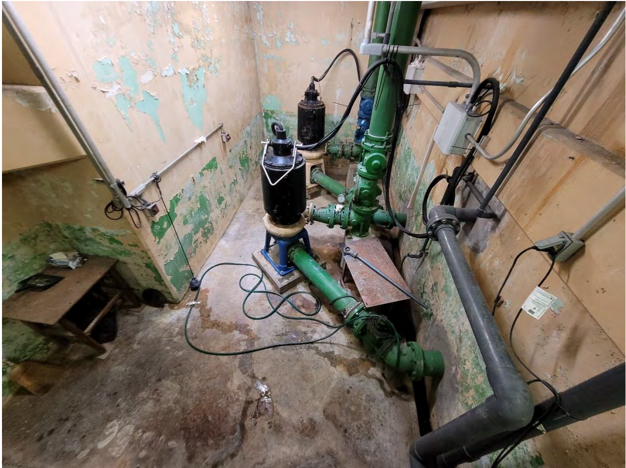
Pumpstation 192: Drywell, Level 2
