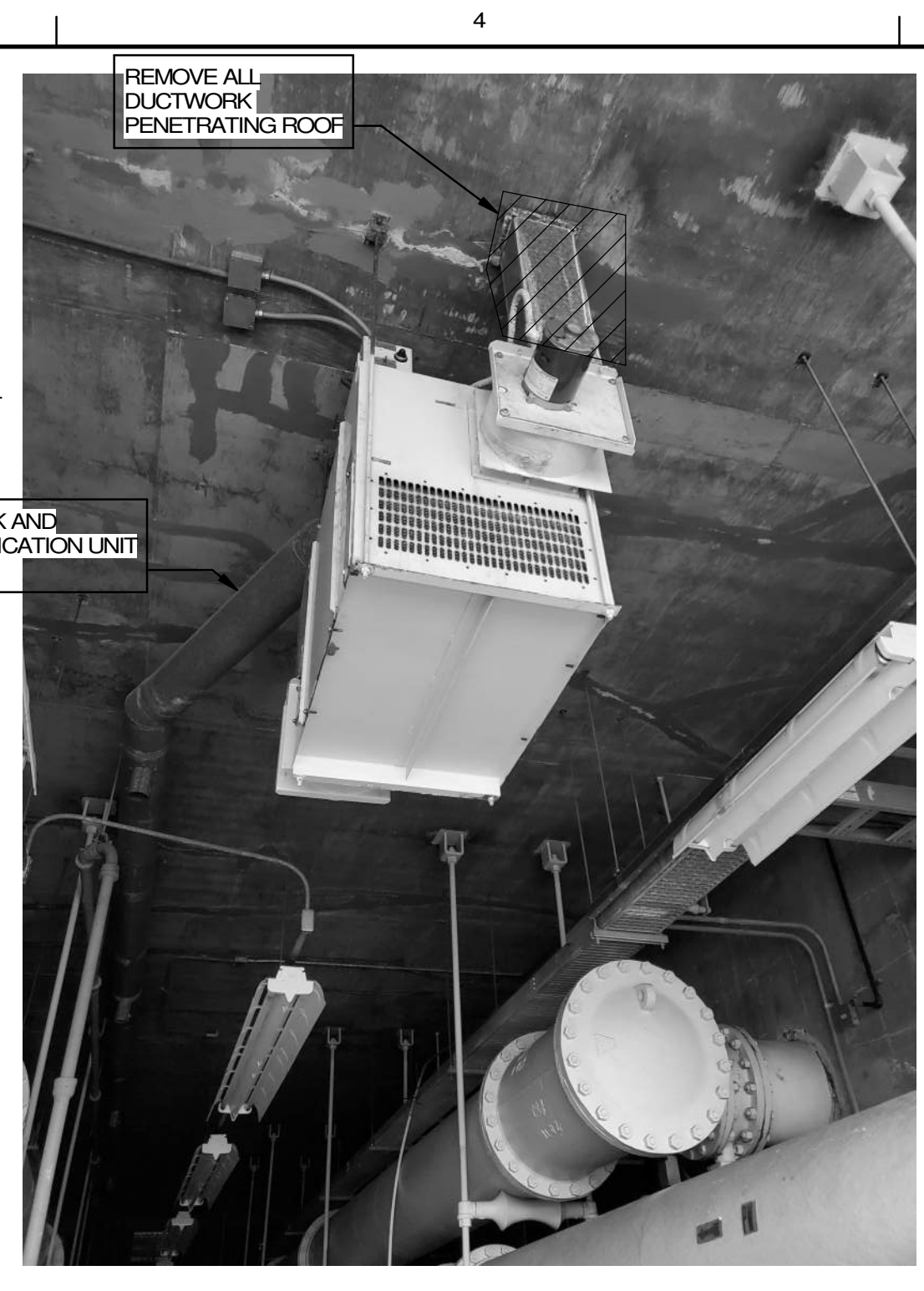
EXISTING DEHUMIDIFICATION UNIT 1/8" = 1'-0"
