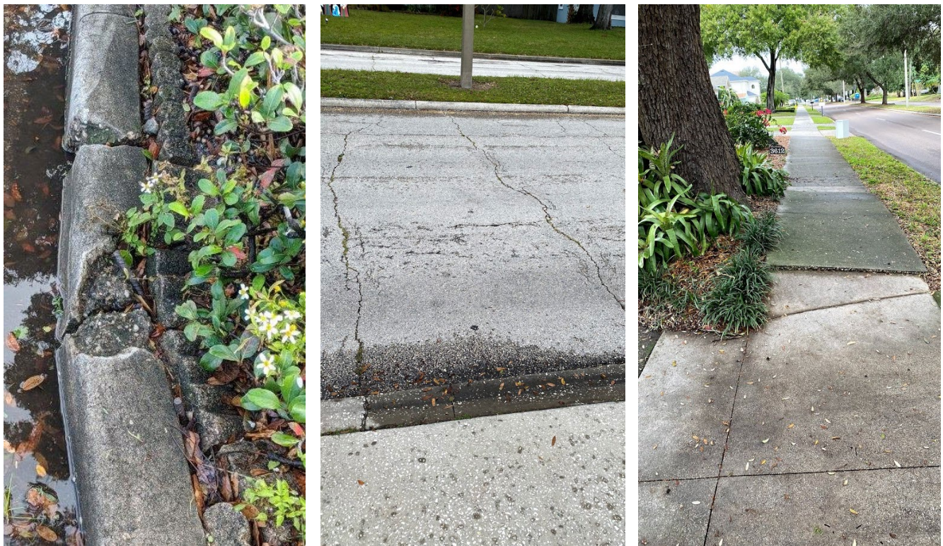
Figure 16: The City will look to rehabilitate the corridor assets; broken curb, pavement failures, and upheaved sidewalks should be evaluated for correction.
