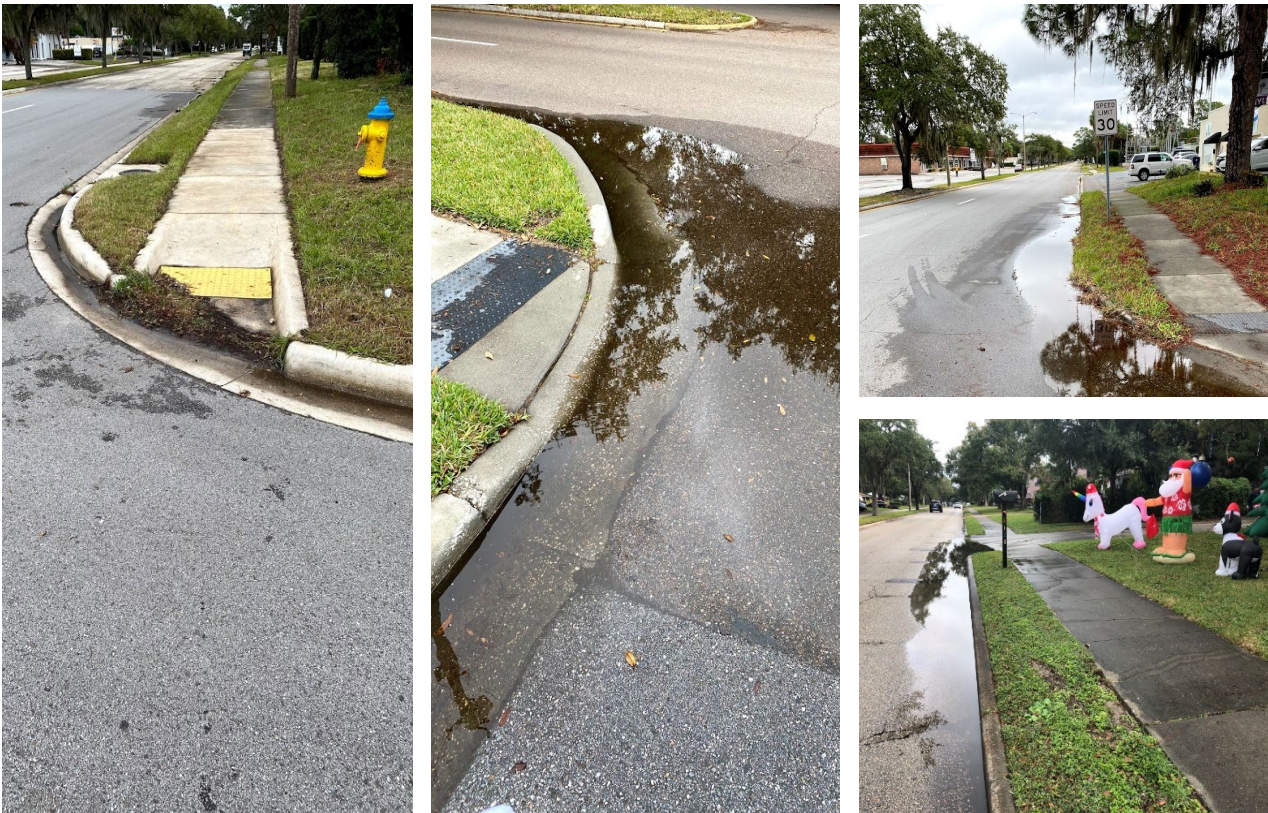
Figure 15: Ponding and sediment in walkways and bikeways create obstacles that reduce the viability of alternate modes
