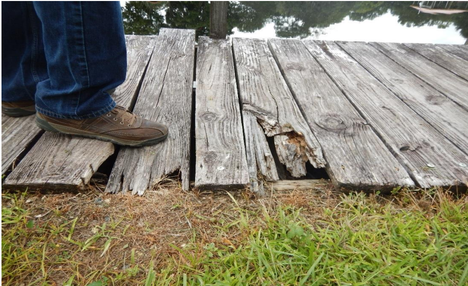
Photo 9-2. Typical decking conditions observed at Rivercrest Park boardwalk showing typical decking conditions.
