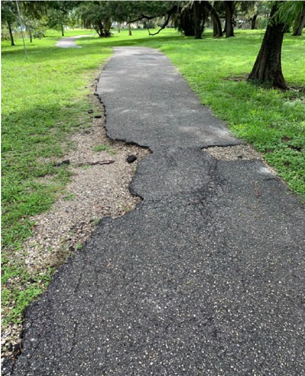
EXHIBIT I: EXISTING TRAIL DAMAGE NEAR THE SEAWALL
