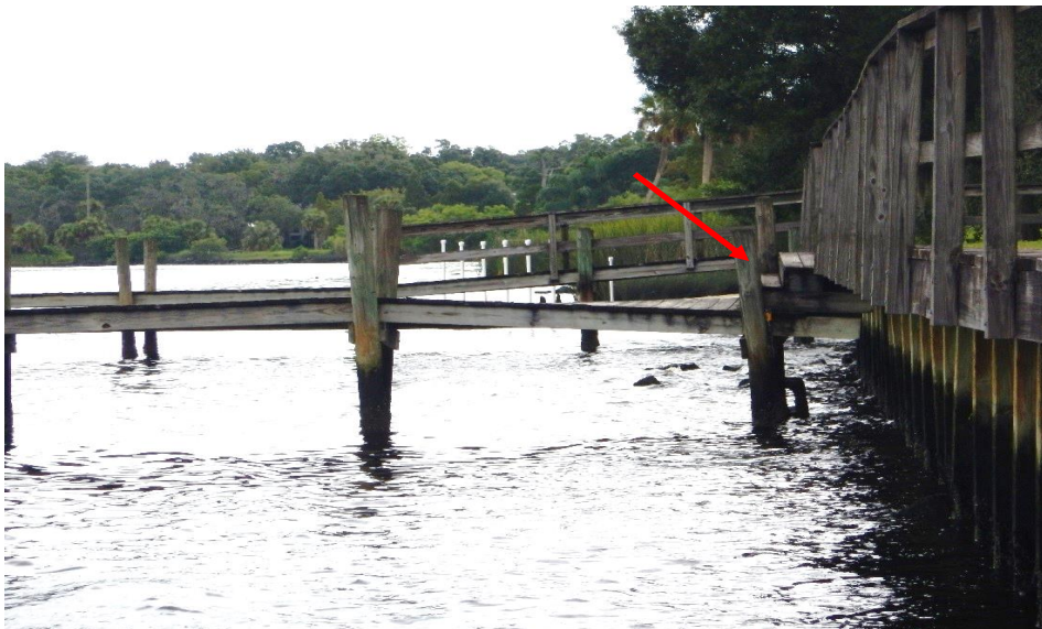
Photo 9-7. Failed pile and settlement at the first bent at Dock 2.
