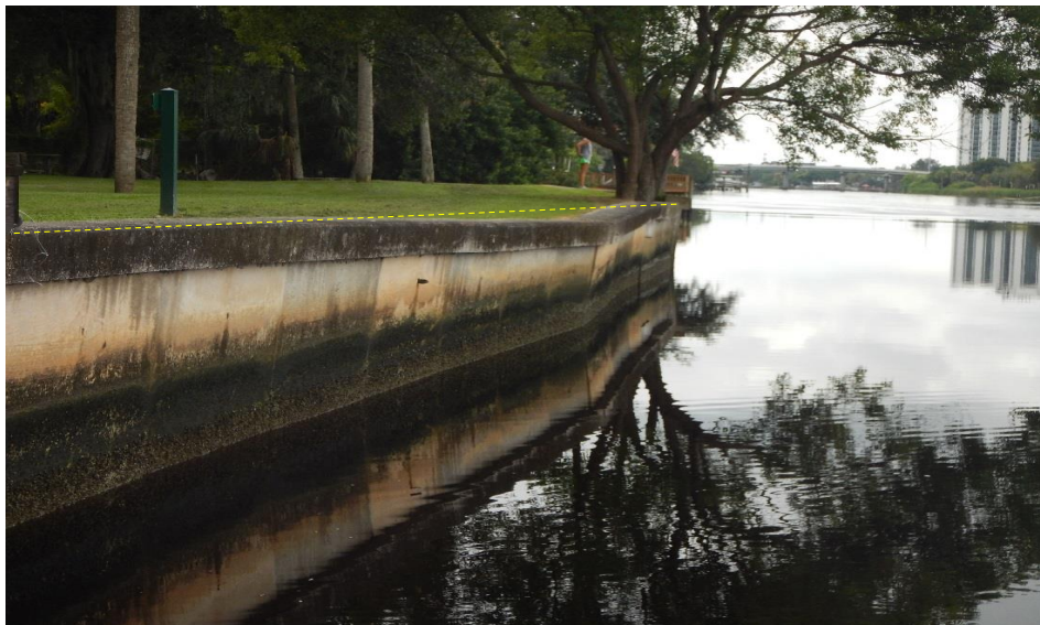
Photo 9-4. Segment in the concrete sheet pile retaining wall leaning over
