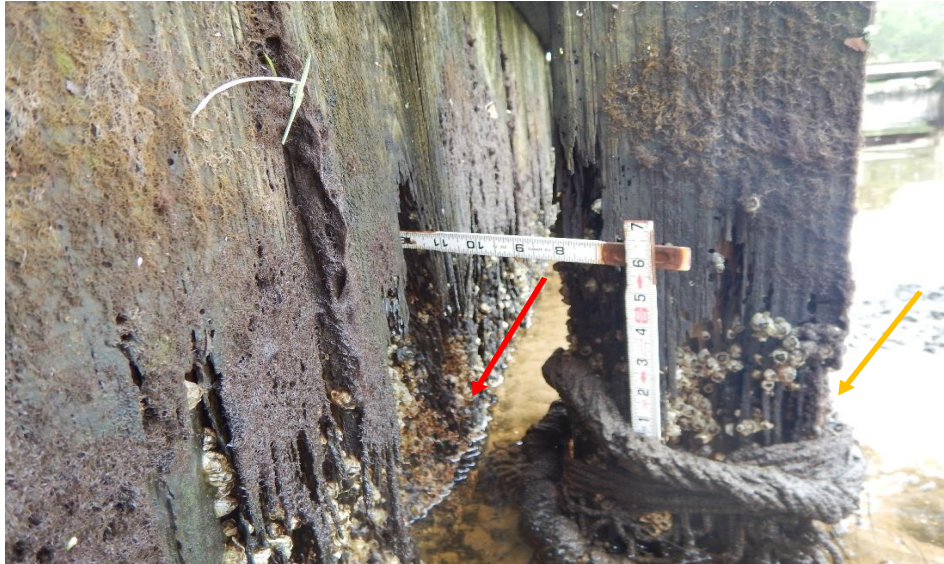
Photo 9-3. Marine borer damage observed on the upstream section of the timber seawall (red arrow) and king piles (yellow arrow) showing a severe damage.
