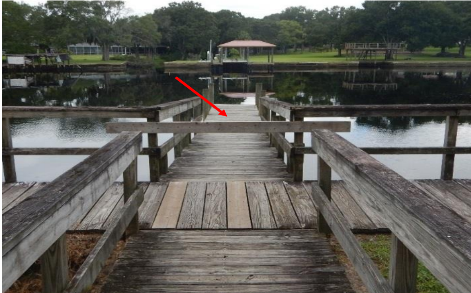
Photo 9-6. Timber Dock 1 at Rivercrest Park has a board across the entrance.
