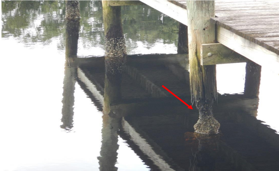
Photo 9-8. Severe marine borer damage (~80% section loss) on timber Dock 3.
