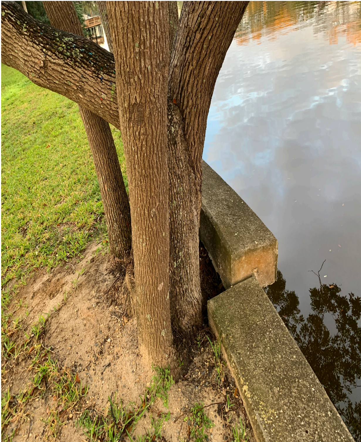
EXHIBIT G: EXISTING CONCRETE SEAWALL DAMAGED BY CAMPHOR TREE
